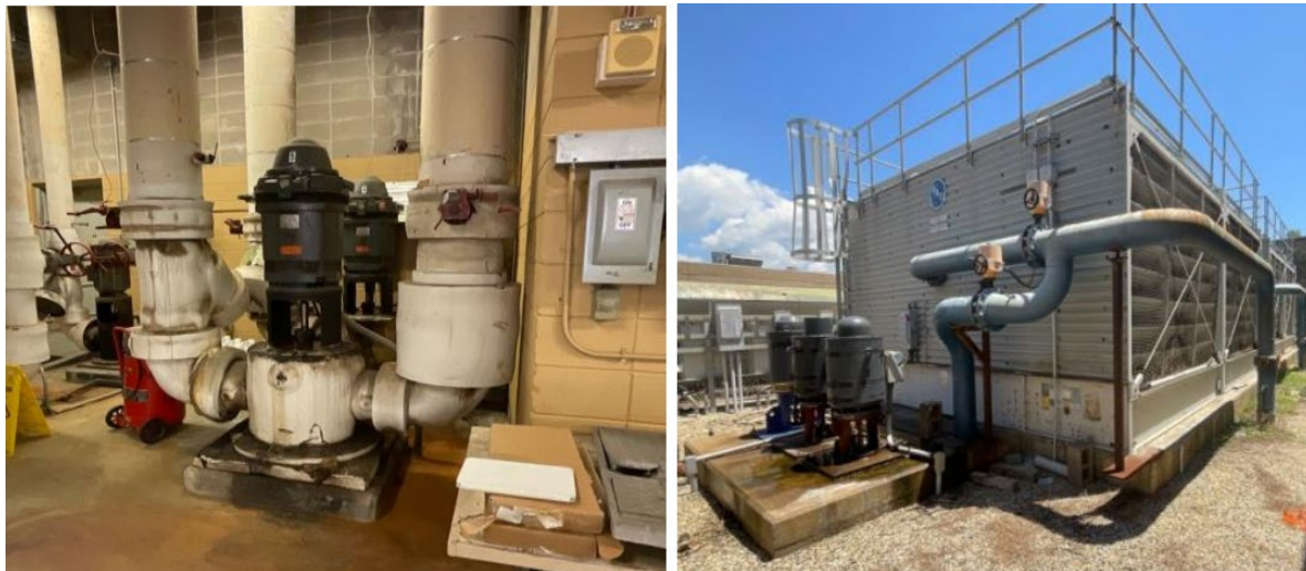
Figure 3 – Plant Pumps & Towers
