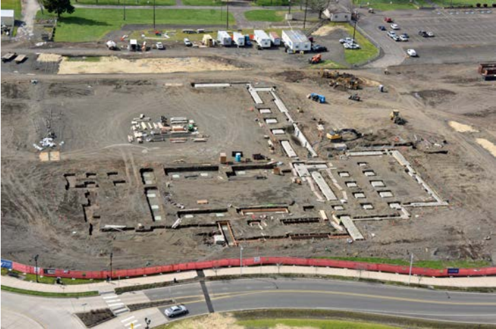
-Footings poured and building footprint takes shape. Area A shown to right, Area B adjacent to NE 34th Ave.
