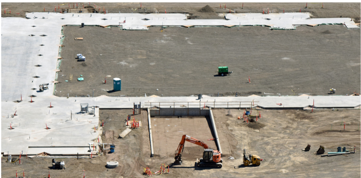
Above: Final preparations to the Loading Dock area are made prior to concrete pour
