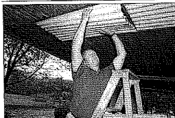
(Mirror photo by Patrick Waksmunski) Sinking Valley Fair President Greg Long repairs a lighting fixture on a building at the fairgrounds. About 90 percent of the event's budget comes from the state, and the current spending plan eliminates the funding.
